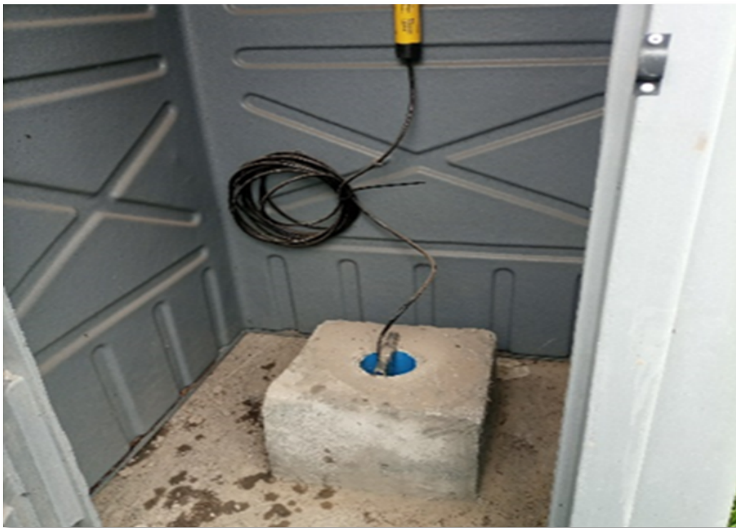
Figure 5: Installed groundwater monitoring device to regulate water level fluctuation and measure salinity of groundwater
